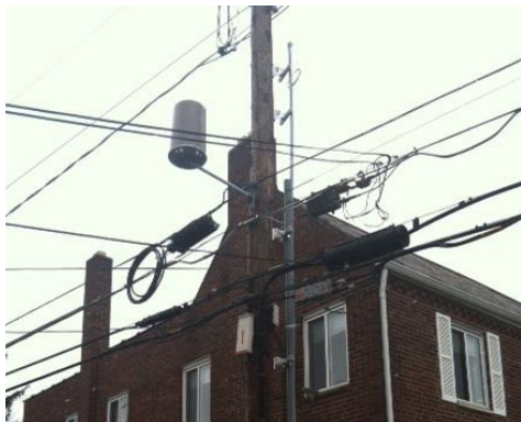
Small cell antenna. Source: Fibertech Networks
