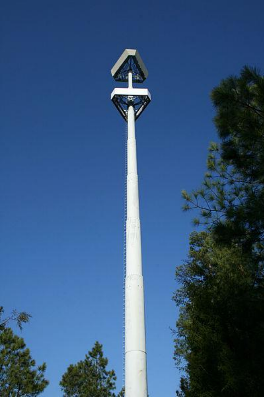
Monopole Tower in Morrisville-Source: Wikimedia
